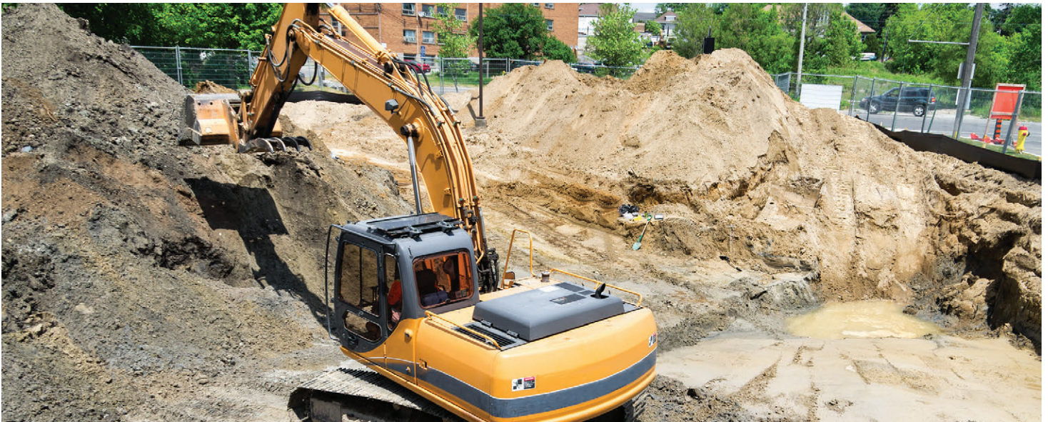
An excavator removing contaminated soil during a redevelopment program. Disposal of PFAS contaminated soil remains largely unregulated in the United States.
