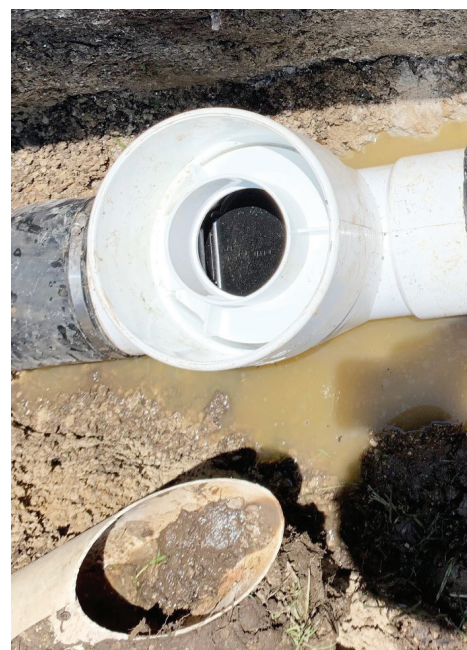
An extendable backflow preventer valve was installed in the sewer's lateral sewer to limit the potential for a siphoning effect.
