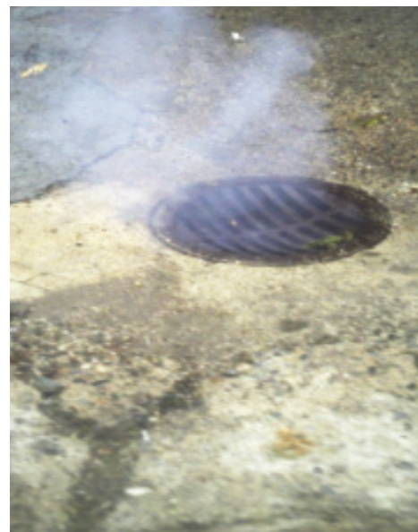
Smoke coming from a floor drain during testing.
