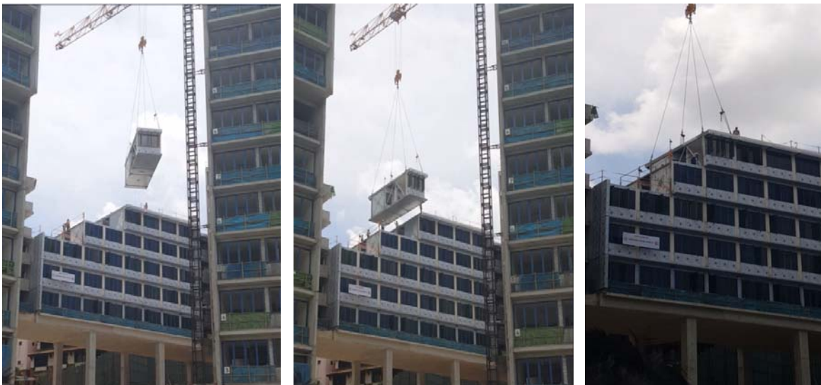
Source: Screenshots taken from video taken during BCAA's seminar 'Prefabricating the Future - A Local PPVC Experience - NTU Nanyang Crescent Hostel'
