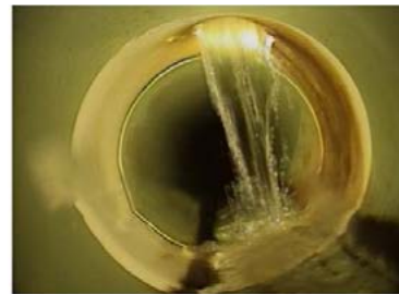
Picture above: Likely illicit sump pump connection discharging inflow of clear water into the sanitary sewer. NEW Water Televising Program 9/6/2018.
